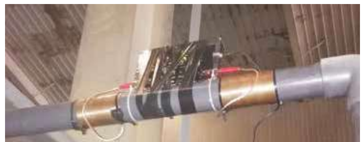
S10 was installed before the reverse osmosis membrane.
