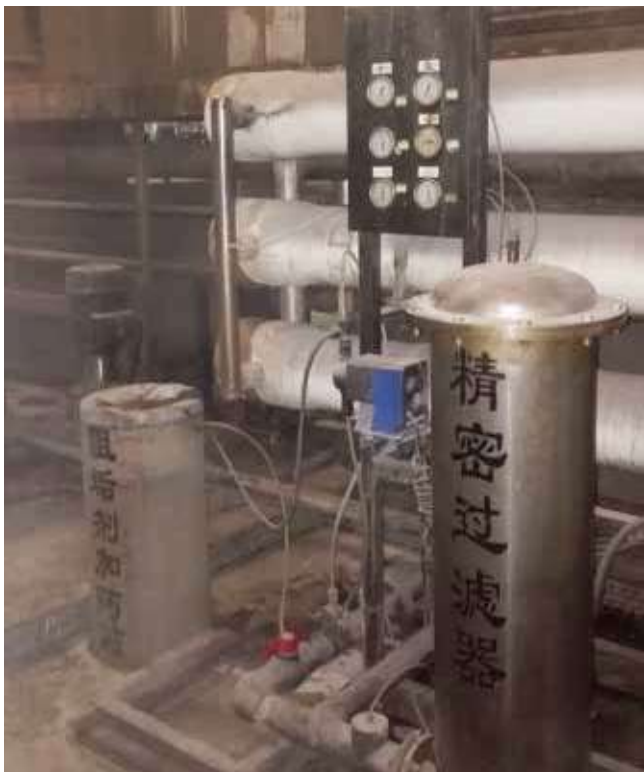
Pure water process equipment.
