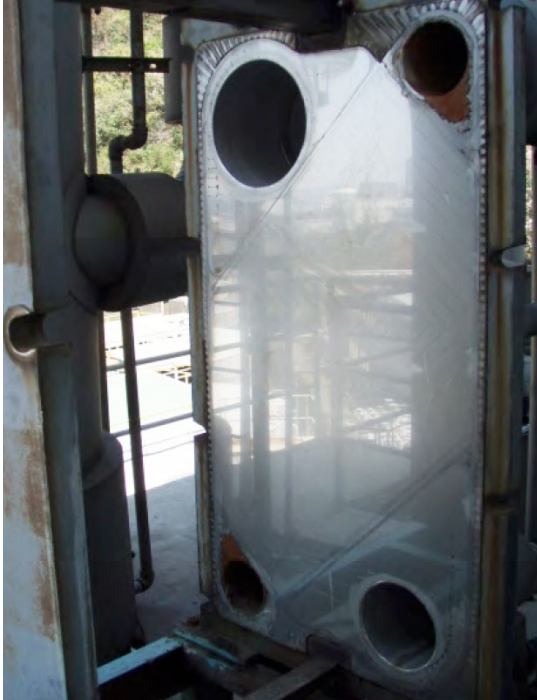
After Vulcan was installed for 9 months: ready open the plate heat exchanger and clean.
