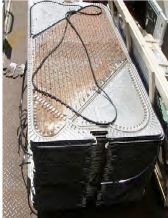
After Vulcan was installed for 9 months: the plate heat exchanger was taken apart for cleaning.
