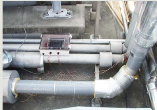
Vulcan S100 installation
